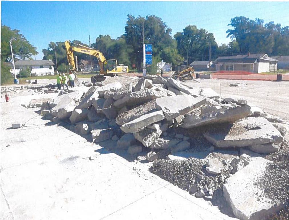
Date: 8/30/2022 Time: 9:47am Direction: Photo by: Robert Mileur Exposure #: 003 Comments: Concrete that covered tank field.
