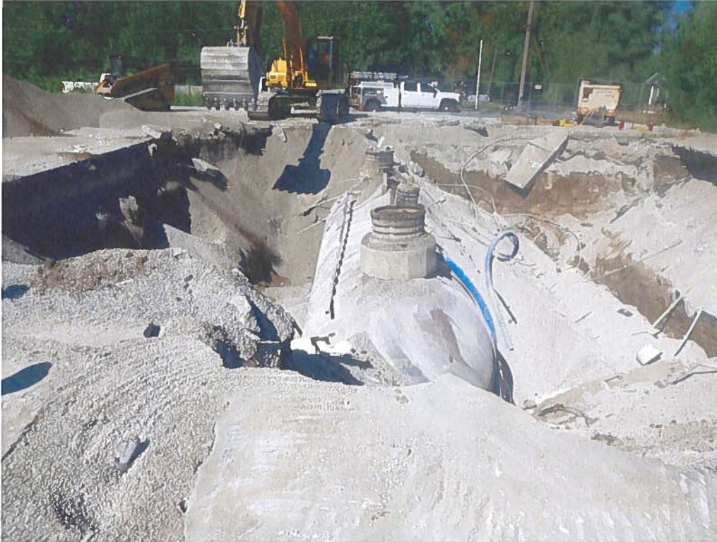
Date: 8/31/2022 Time: 10:32am Direction: W Photo by: Robert Mileur Exposure #: 011 Comments: Getting closer to removing UST.
