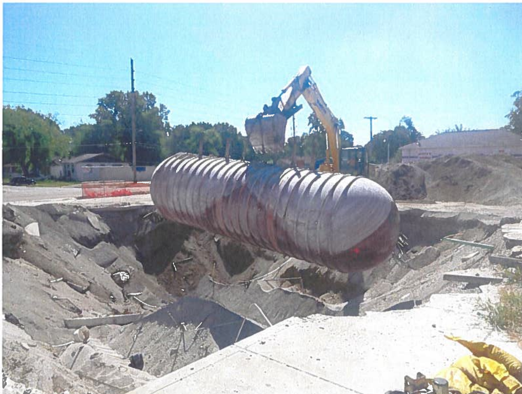
Date: 8/31/2022 Time: 11:18am Direction: SE Photo by: Robert Mileur Exposure #: 012 Comments: Removing second UST from tank field.
